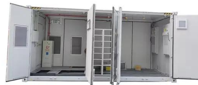
1075KW HH ESS
