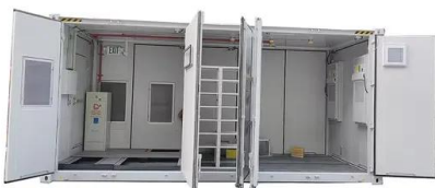
1075KW HH ESS
